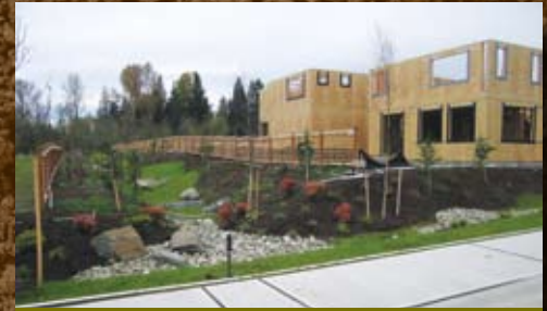
At Shamrock Heights, Cam West Development combines a traditional feel with innovative stormwater methods. Reuse of high-quality site soils plus mulching support a vibrant landscape.
